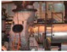
E148 expander hot mechanical spin test (Olean, NY, USA). Dresser-Rand has invested in the most advanced testing capabilities in the industry, and maintains world-class test facilities in Olean; and in Le Havre, France.
